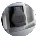
Power outlet for electric tool
